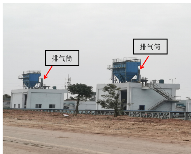
DJ1、DJ2 转运站粉尘排气筒
